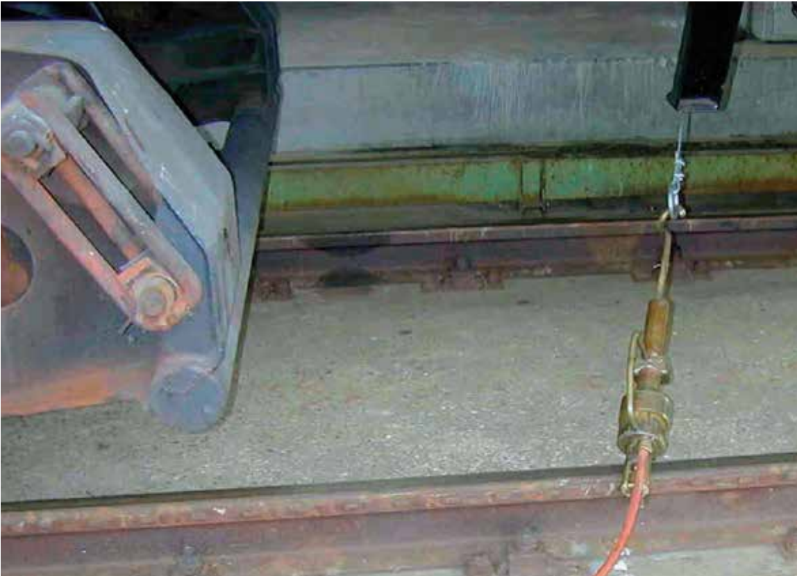
Fig. 9 Rail hook combined with a remote control, which closes the bottom valve if activated. This example shows only the set up for liquefied gas railcars.
